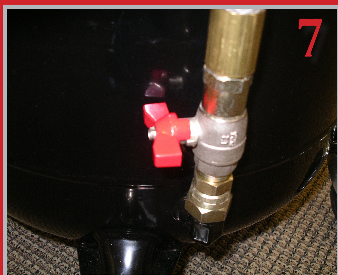
7 Close material outlet shut-off valve at the base of the drain.
